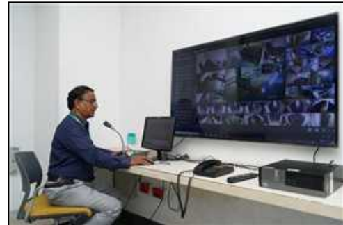
Learning Centre - CCTV Monitoring
