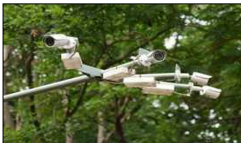
Campus - CCTV Surveillance
